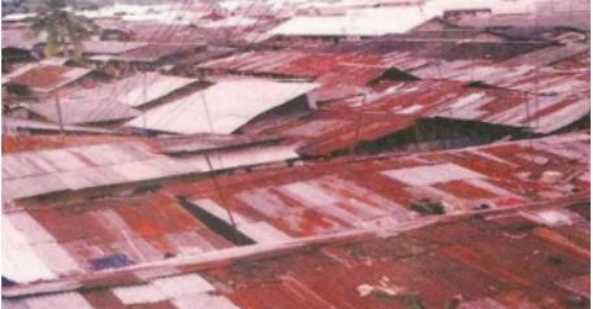
Figure 3 CORRODED BUILDING ROOF WITH ACID RAIN IN THE STUDY AREA
