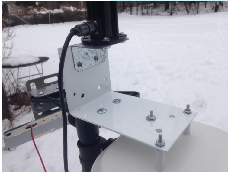
Figure 12: Anemometer and radiation shield bracket mounts.
